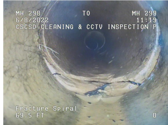
Example 4: Spiral Crack
