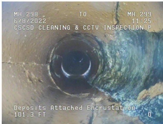
Example 3: Encrustation Deposits/Infiltration Stain
