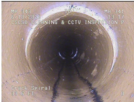
Example 1: Spiral Crack
