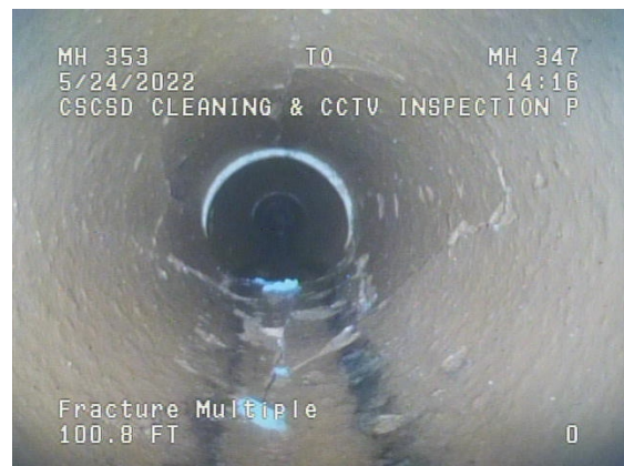
Example 6: Multiple Fractures
