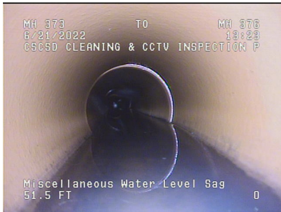
Example 9: Pipe Sag
